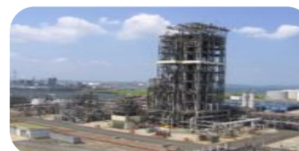
Condensate Splitter Unit (CSU)
